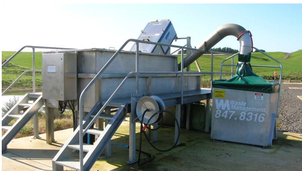
Figure 4-2 Covering of Screenings
