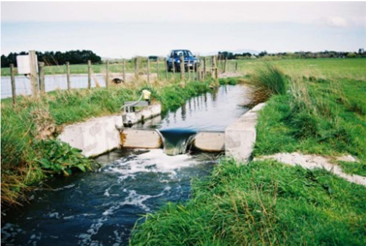
Figure 2-7 V-notch weir with ultrasonic depth measurement on pond effluent
