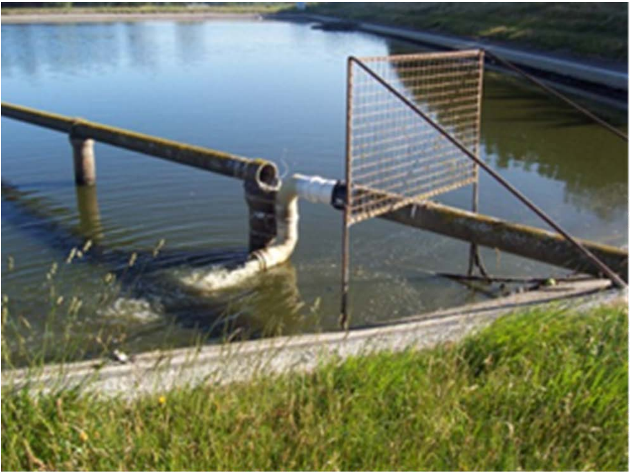
Figure 2-2 Modifications to Pond inlet – to provide jet attachment to the embankment wall
