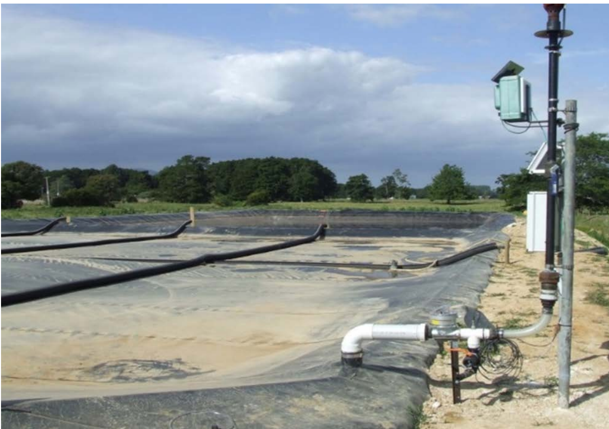
Figure 2-1 Covered Anaerobic Pond with Biogas Flare
