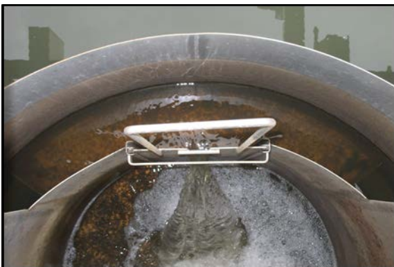
Figure 3-7 Flow Control Weir
